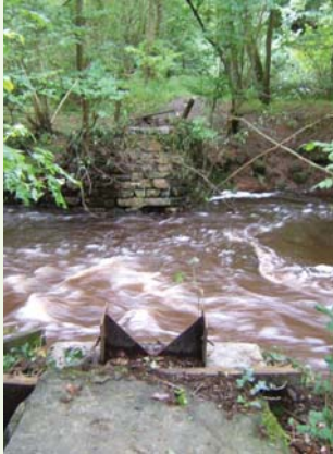
Flood Damage at May Beck
