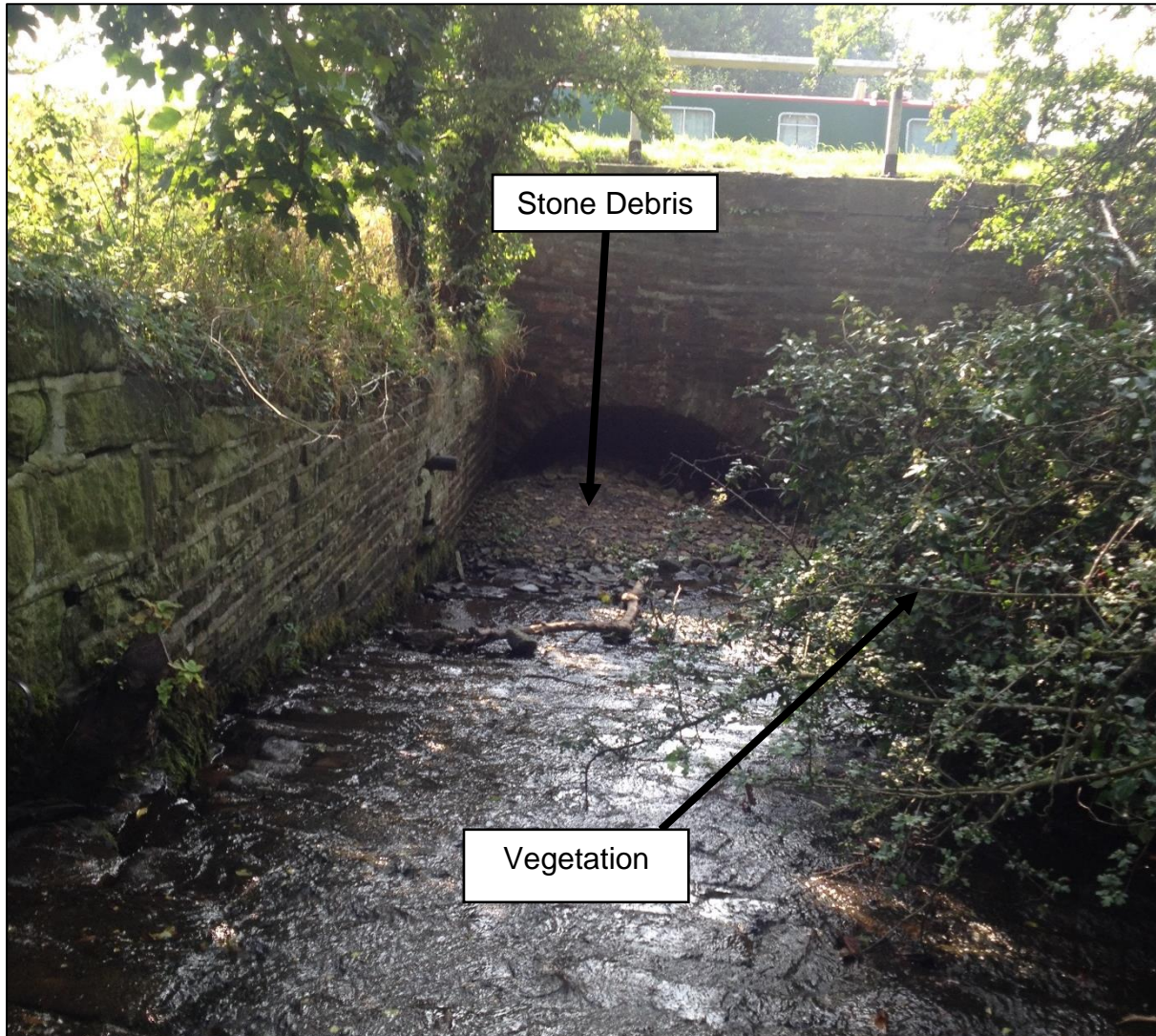
Figure 4.7 Photograph showing deposits in canal
