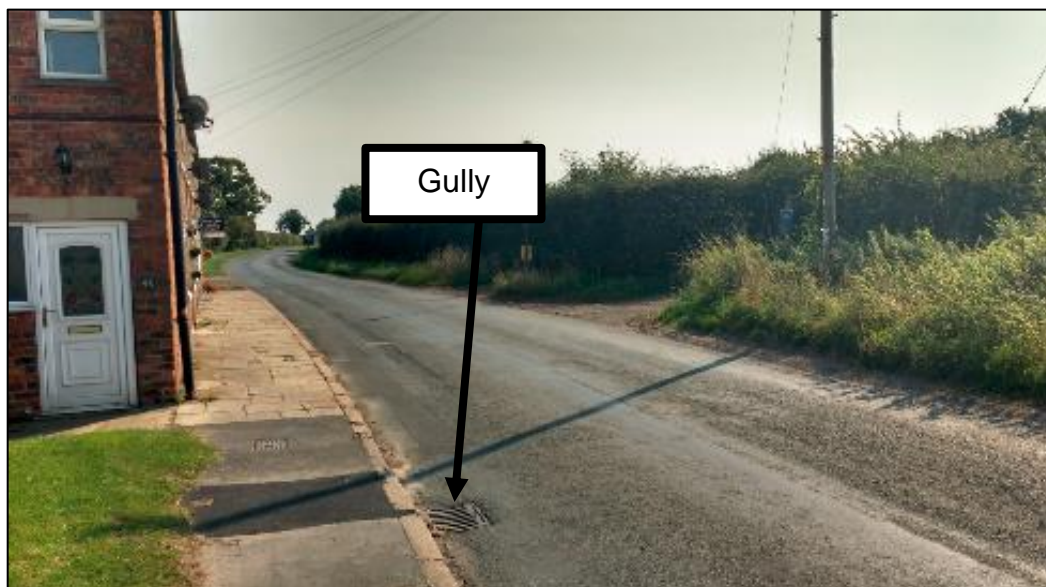
Figure 2.7 Road Gully on Marston Road outside New Row Cottages
