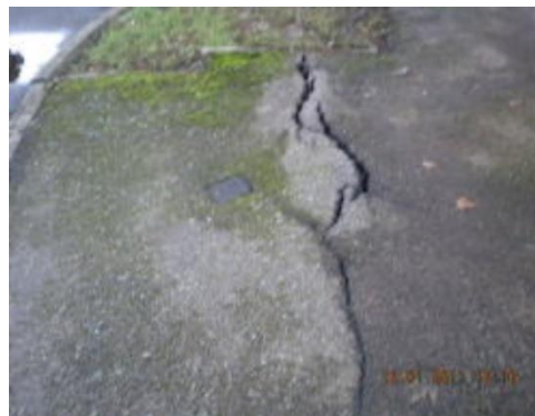
Tree root damage to footway
