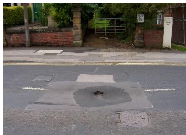
Depression in centre of road
