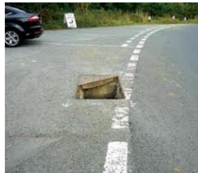
Missing Inspection cover
