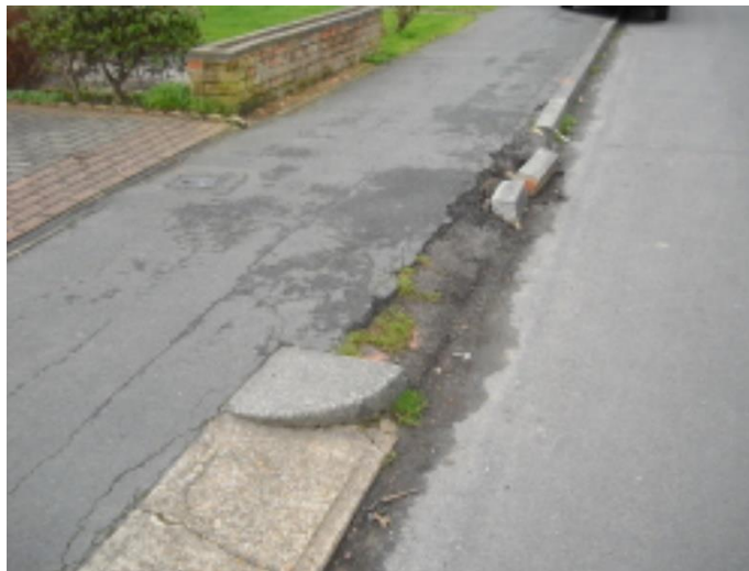
Kerb misaligned horizontally
