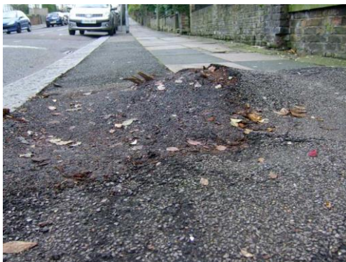
Tree root damage to footway
