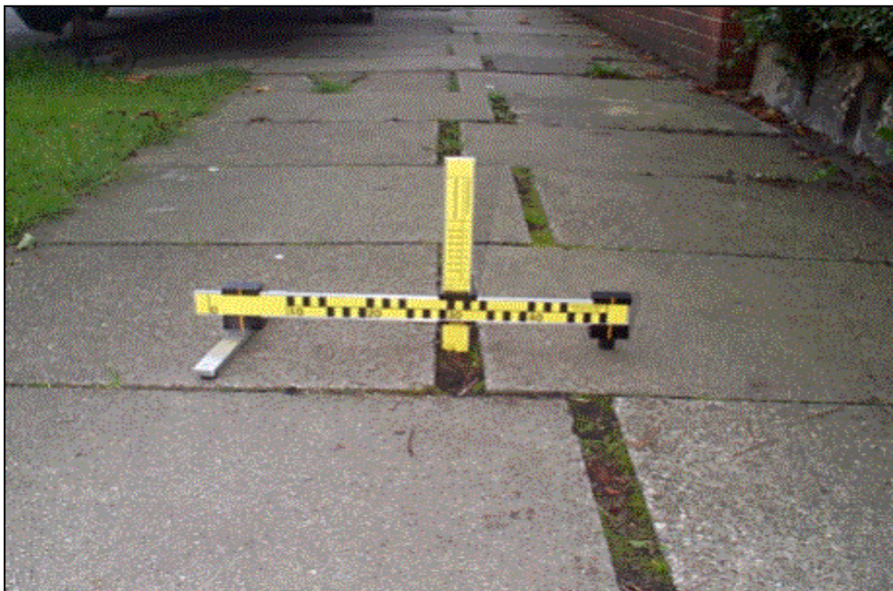
Open joint between paving stones
