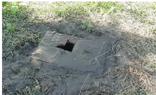
Broken Inspection cover
