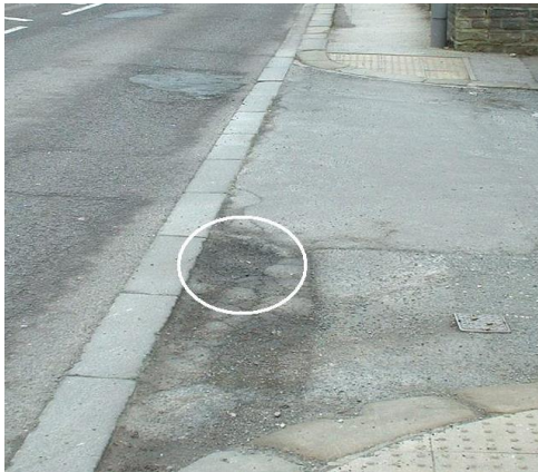
Potholes in pedestrian crossing of side road
