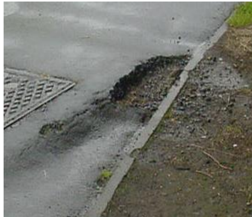
Pothole in footway exposing unbound material
