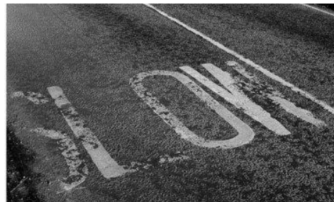
Approx 30% faded markings
