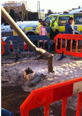
Damaged in RTA
