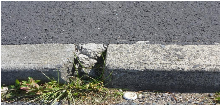
Gap between kerbs
