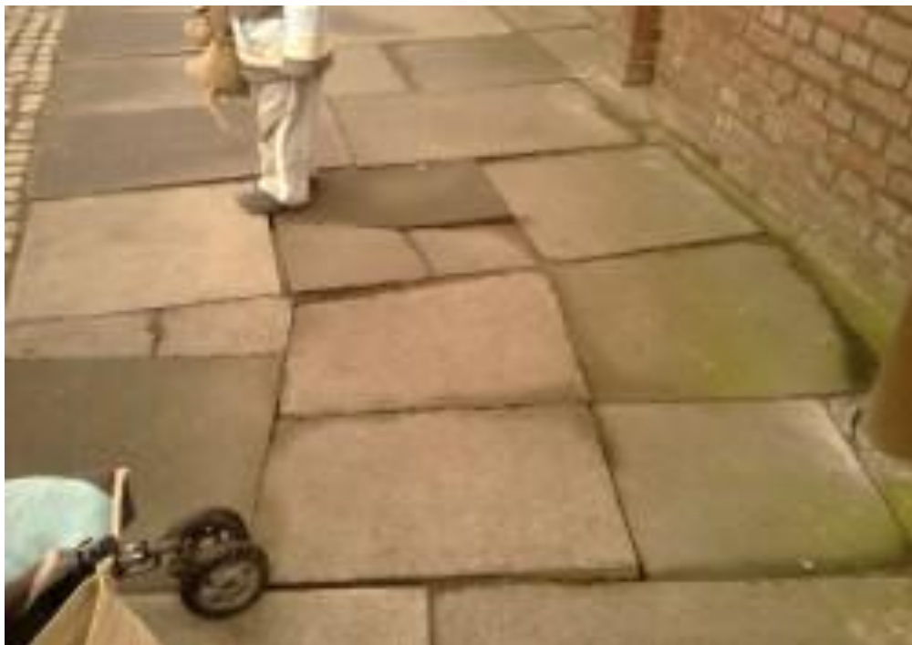
Loose paving stones
