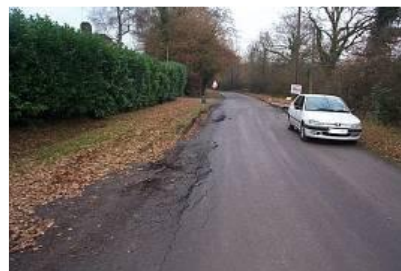
Depression and heave along edge of road
