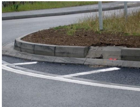
Kerb misaligned horizontally away from carriageway
