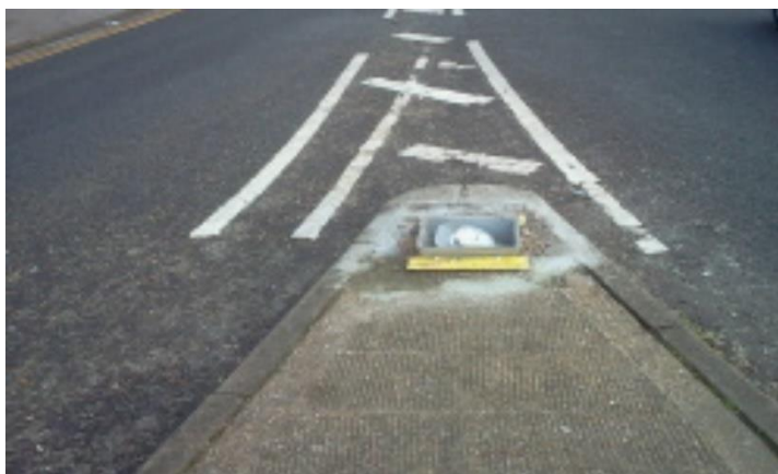
Missing keep left bollard
