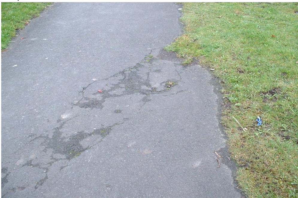
Subsidence in footway
