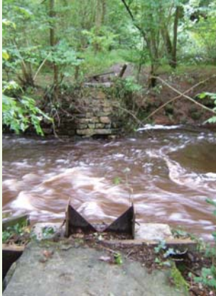
Flood Damage at May Beck
