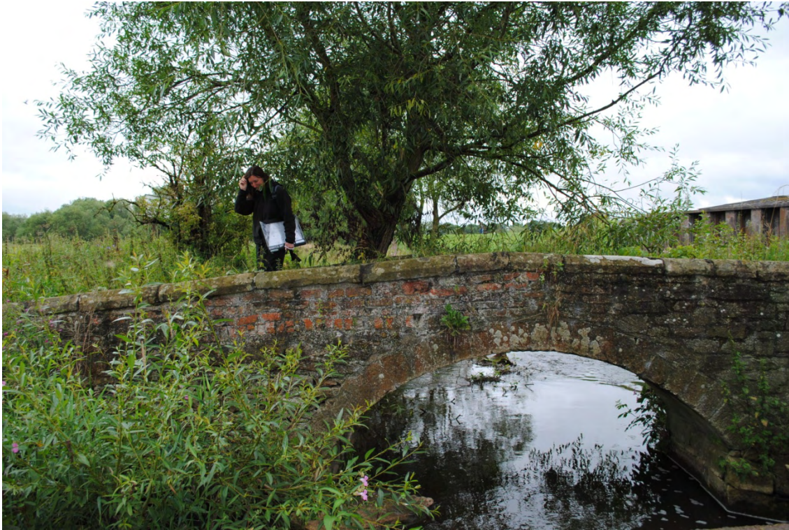
Photo: Lan 1.1.4a Clow Beck Pack Horse Bridge near Monk End Farm (grade II)
