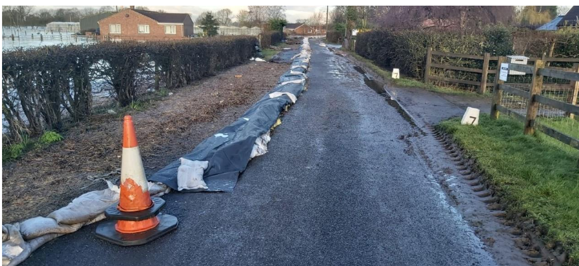
Figure 19: West Bank Visqueen and Rubble Defence
