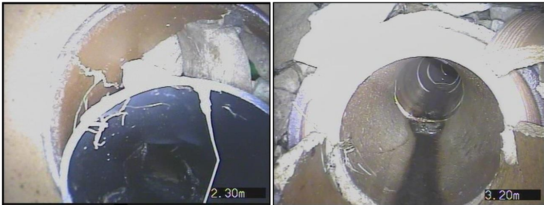
Figure 3.7 Photographs demonstrating damage to the culverts under the A169. (Source: NYCC)
