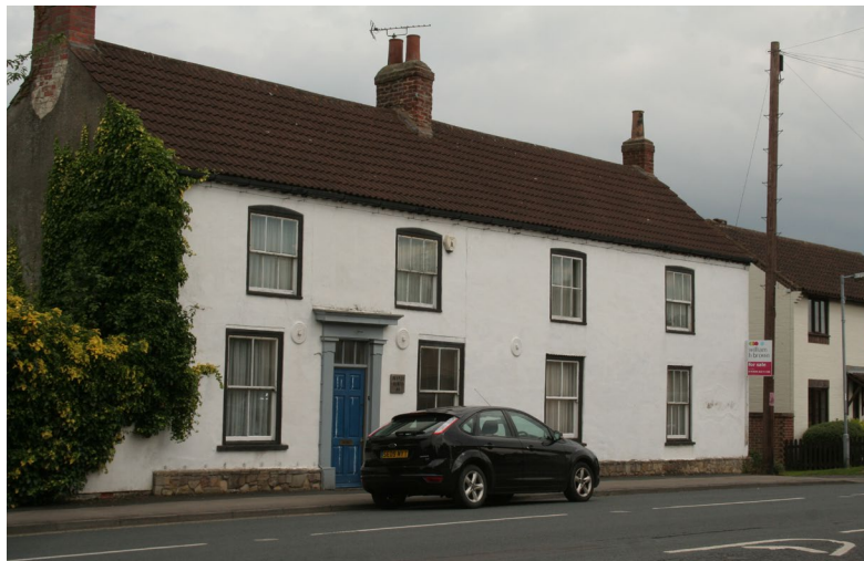
Reconstituted stone pantiles on an otherwise very characterful former public house on Main Street (Drovers Cottage). Note the surviving timber sash windows
