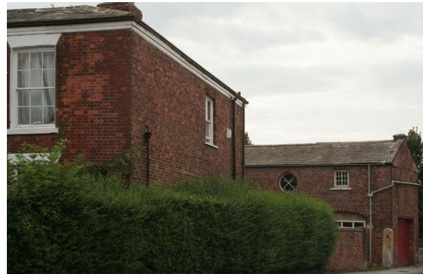
Hedge boundary and brick wall at the Grade II listed Red House on Silver Street illustrating the importance of out buildings to the character and appearance of the conservation area.
