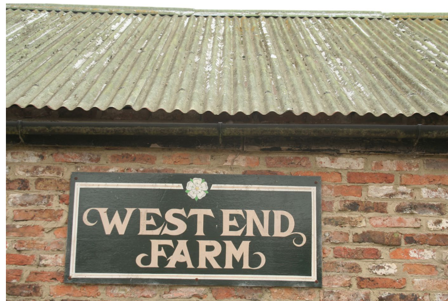
West End Farm nameplate. Note the corrugated iron roof, presumably replacing earlier clay pantiles
