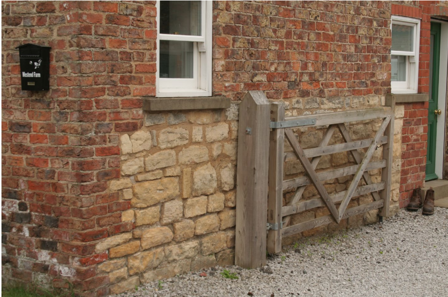
Detail of the main farmhouse at West End farm showing the magnesian limestone walling that may be part of an earlier building
