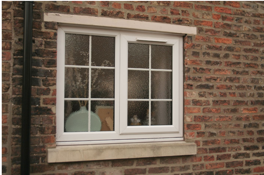
Detail of a uPVC window replacement that lacks any reference to the original timber sash
