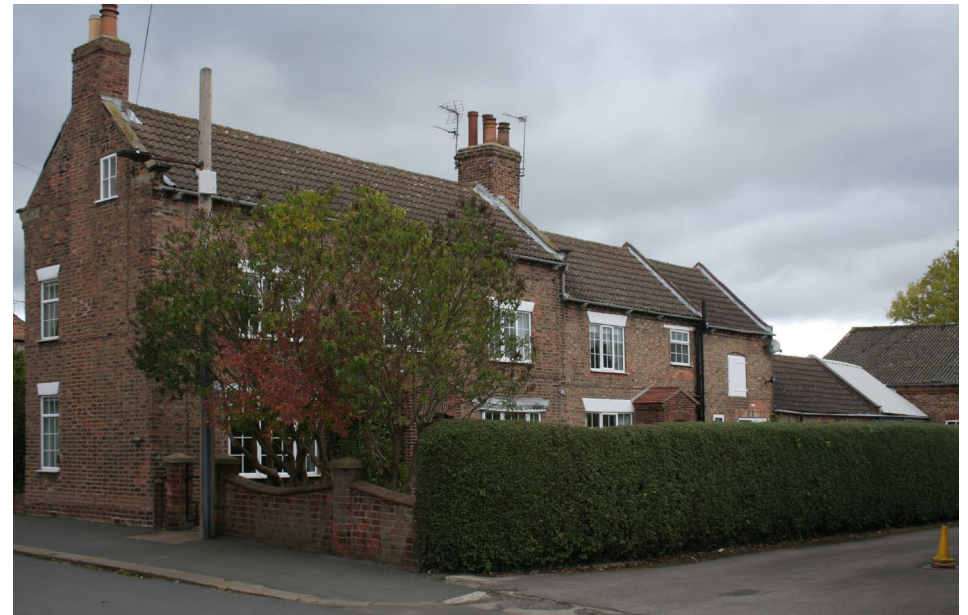
Former early 19th century farm, number 9 Wistowgate showing impact of the use of reconstituted stone pantiles that have replaced original traditional clay pantiles
