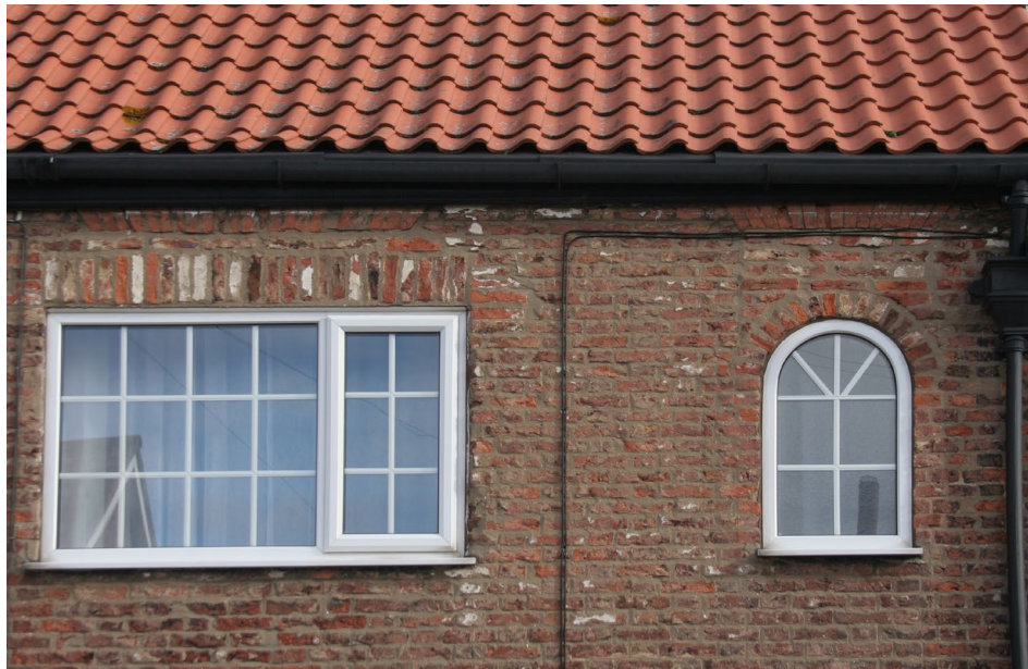
Example of upvc window replacements on an undesignated early 19th century building on Rythergate
