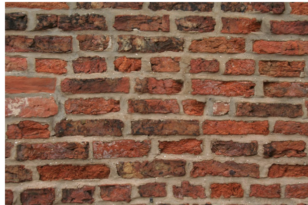
An example of local late 18th century hand made brick. Note the relatively rough pointing.
