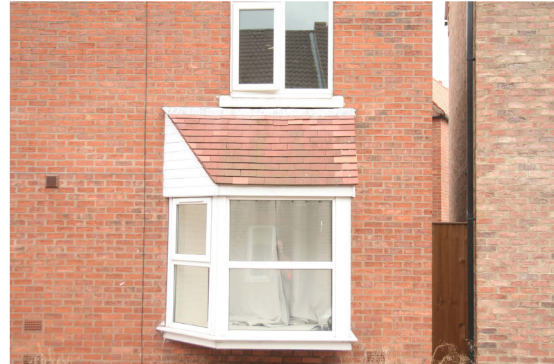
Late 20th century projecting bay at Friendship Court fronting onto Millgate adding an incongruous contemporary element into the historic street scene
