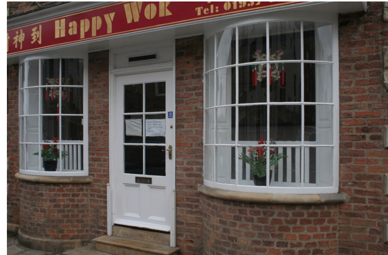
Poor reconstruction of a shop front on an historic but non-designated building on High Street
