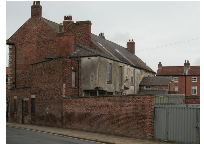
A Brick boundary wall on Westgate marking the rear of the Grade II listed 49 Kirkgate
