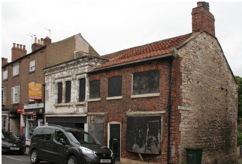
Brick facing on an earlier limestone construction at 24 Kirkgate. Note the dilapidation on this and the neighbouring building
