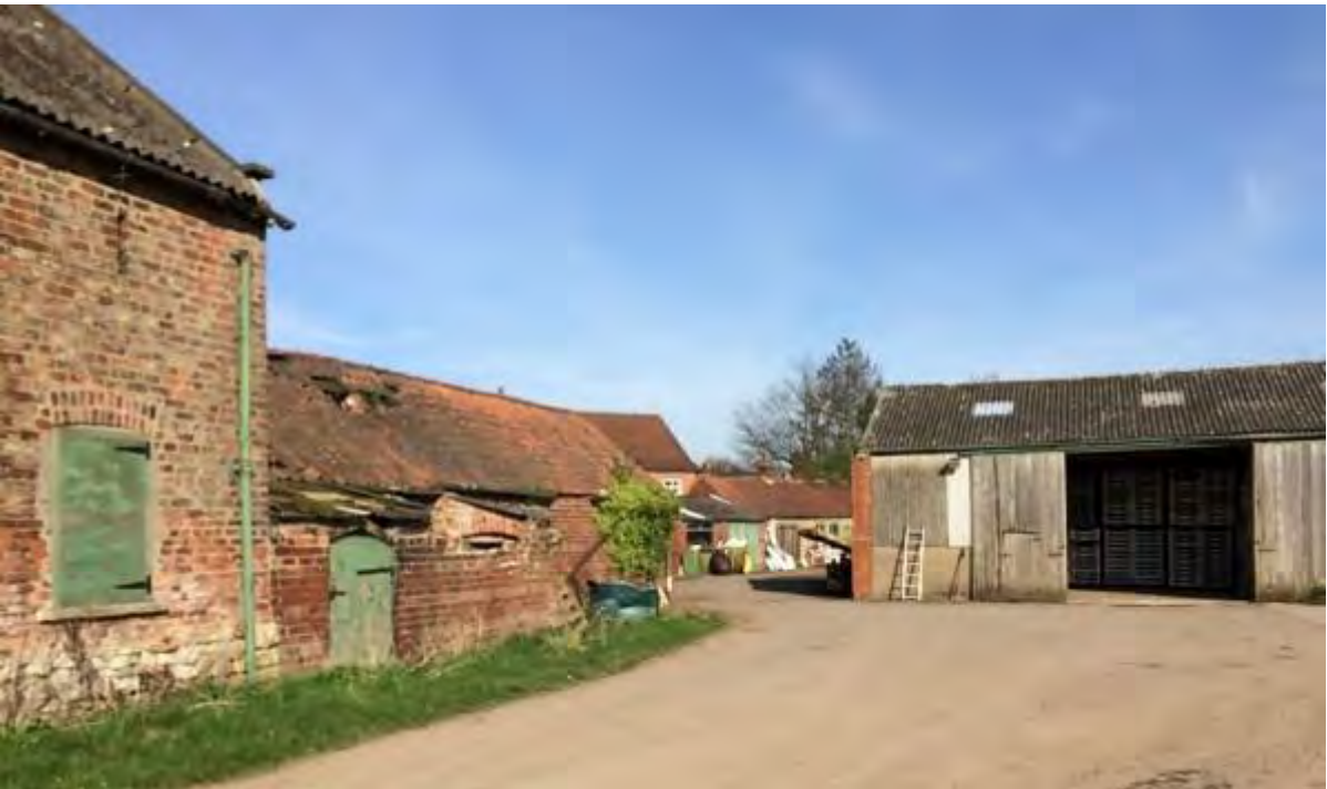
Above: Photo 3 - Farm buildings (Garth Lodge behind), Source: Archaeology & Built Heritage Assessment by Pegasus Group, dated May 2017 in relation to planning application 2017/0526/OUTM. Range of buildings to left date from 1845-8 or earlier.
