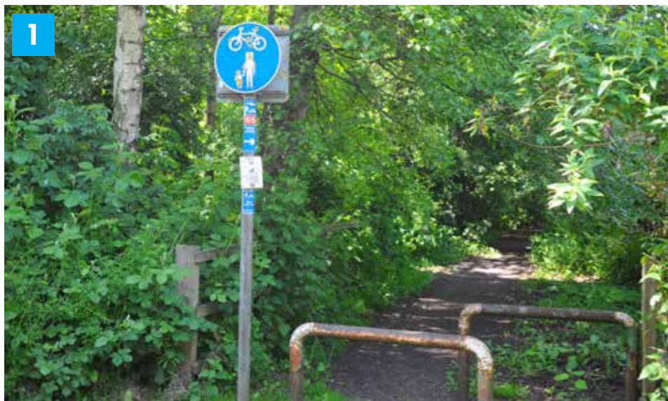
1 Link to Trans Pennine Trail (TPT) from Barlby Road. Some refurbishment of signage and fixtures required to improve visual quality
