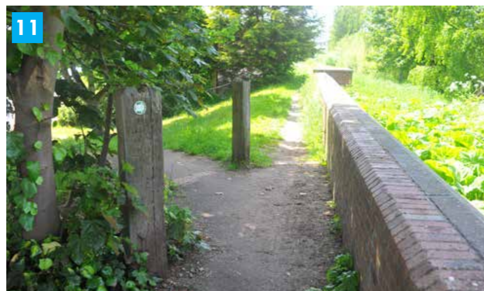
Former landscaped access requires refurbishment/re-design
