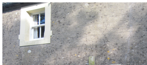
Smooth render lined out to imitate stonework
