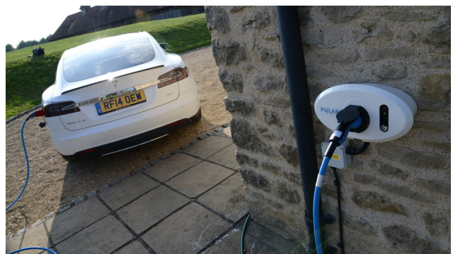
EV plug-in charge point
