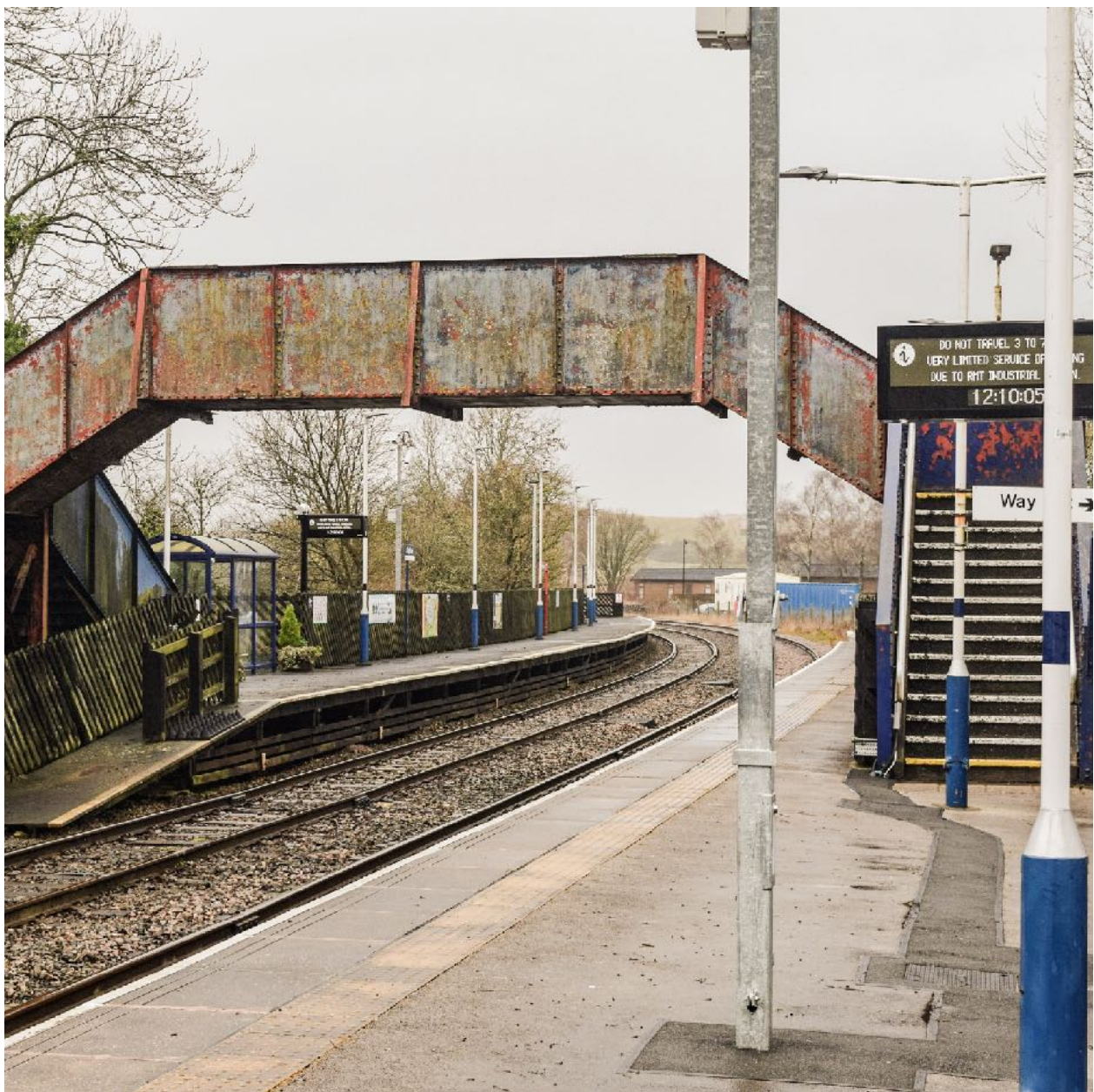
Footbridge across Clapham Station. There is no ramp and the westbound platform towards Morecambe can only be accessed via the footbridge
