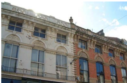
Painting of the property facade on the left, masks interesting architectural detail and destroys the unity of this terrace on James Street.
