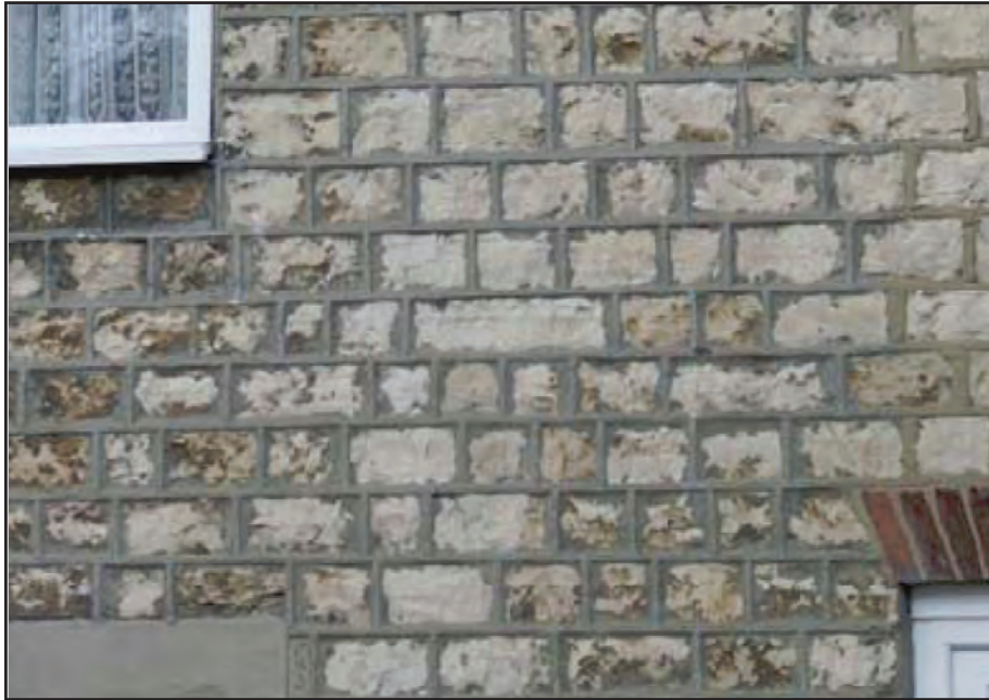
Figure 20: Inappropriate cement mortar finished to a strap profile not only adversely affects the appearance of the building but will also lead to accelerated erosion of the stone.
