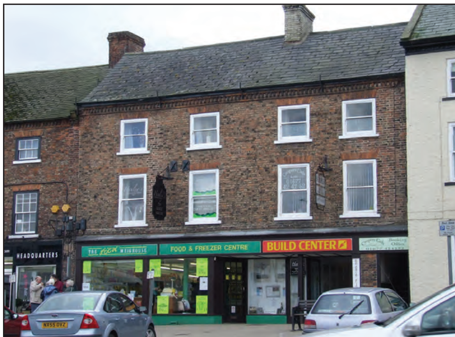
Figure 5: There is no visual support to the upper floors from this 1960's shop front.
