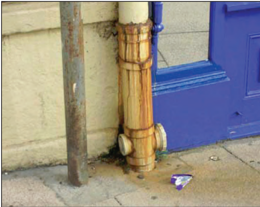
Figure 19: Base of original cast iron rainwater pipe repaired with inappropriate plastic section.
