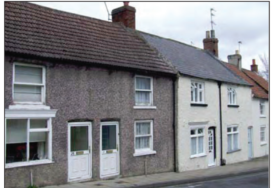
Figure 22: Inappropriate cement render with “pebble dash” finish.
