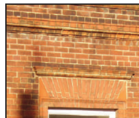
Inappropriate brick selection
