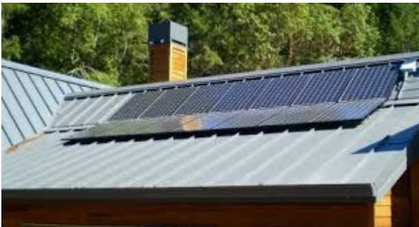
Figure 5.1 Photovoltaic cells on a standing seam roof
